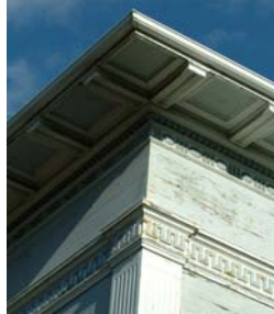
Freize with modillion block with Greek key decoration below it under the eaves.
